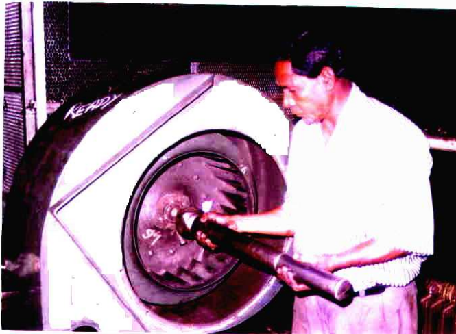
Figure 3.6 Wrong fitment of Impeller
