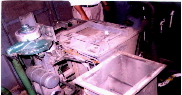
Figure 3.4 Motor foundation and MVMT Duct in loco
