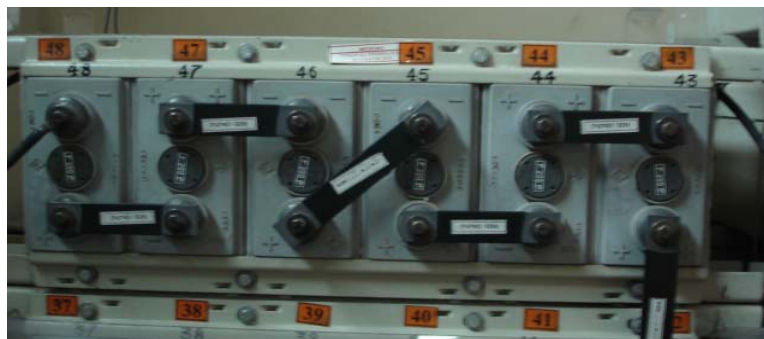
Fig. 2.10 : VRLA battery bank
