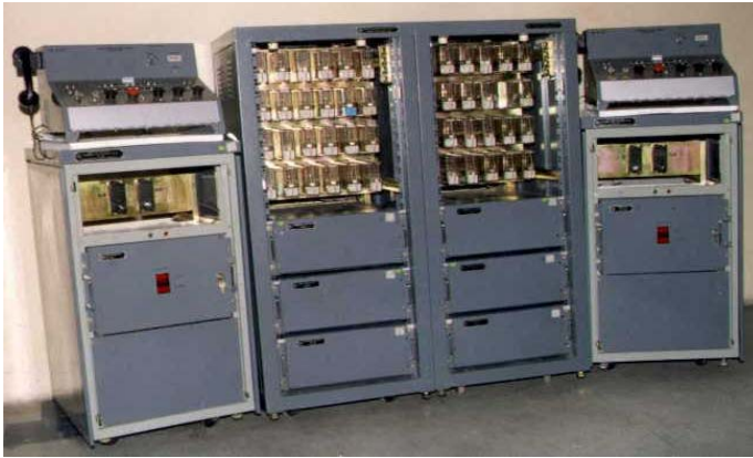
Multiplexer & Prewired Relay Rack Fig. No. 3
