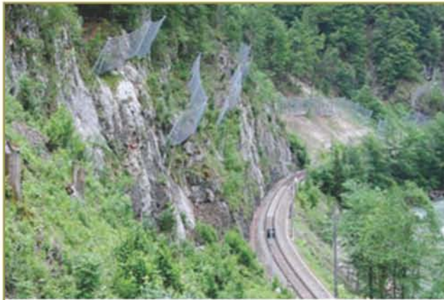
Fig-5: Flexible Rockfall Barrier
